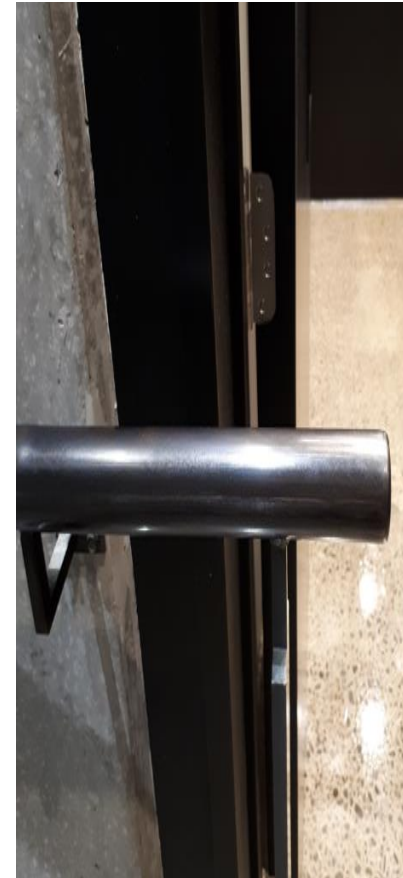
Photo 6 – Level 1 Stairway Balustrade Protrudes
