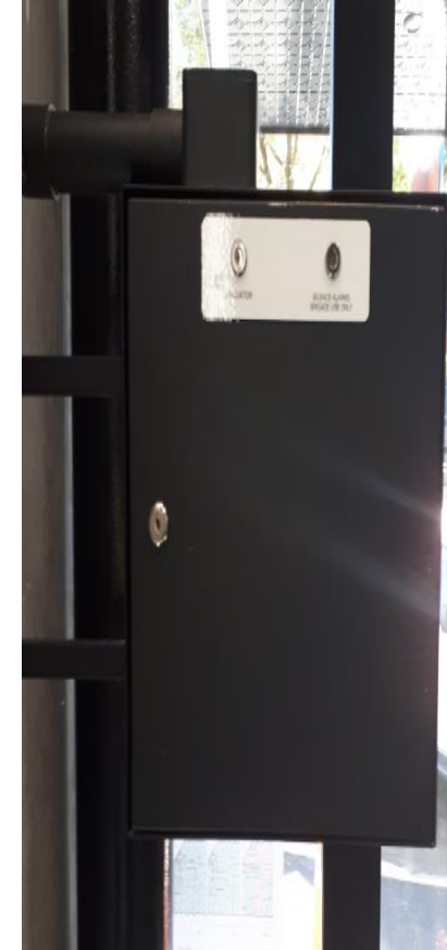
Photo 4 – Entrance Foyer Black Alarm Box
